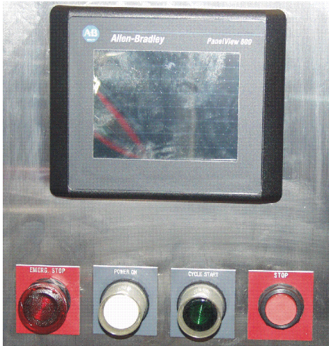
Figure 11 Operator's Control Panel
